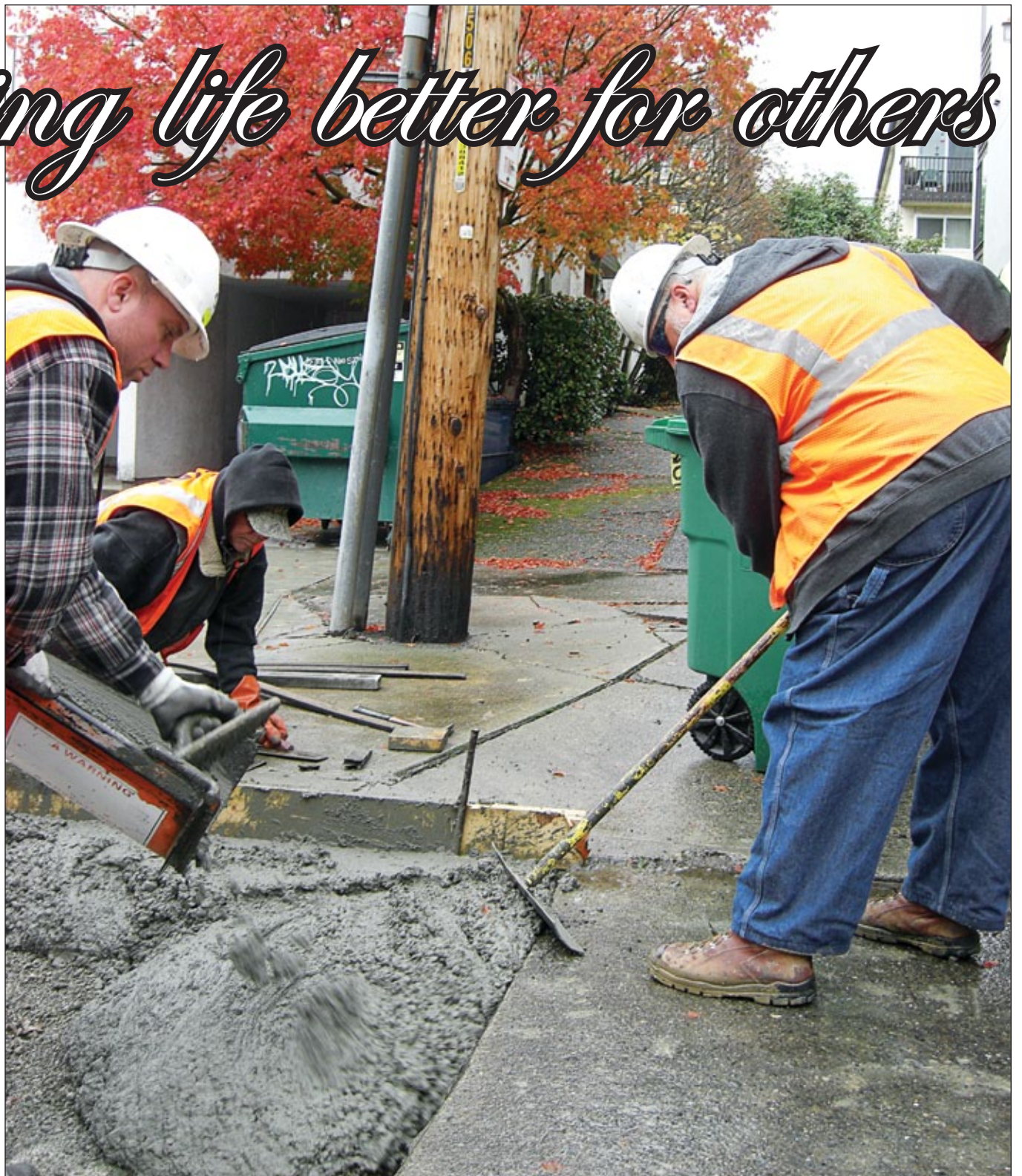
Seattle City worker Jack Aubrey, right, helps build a concrete street panel. With him are fellow workers Mike Houston and Pete Hagan.
