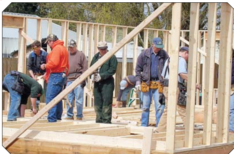
Members of Local 176-SW join other volunteers in building a house for Habitat for Humanity. In the orange jacket is member Steve Huizinga.
